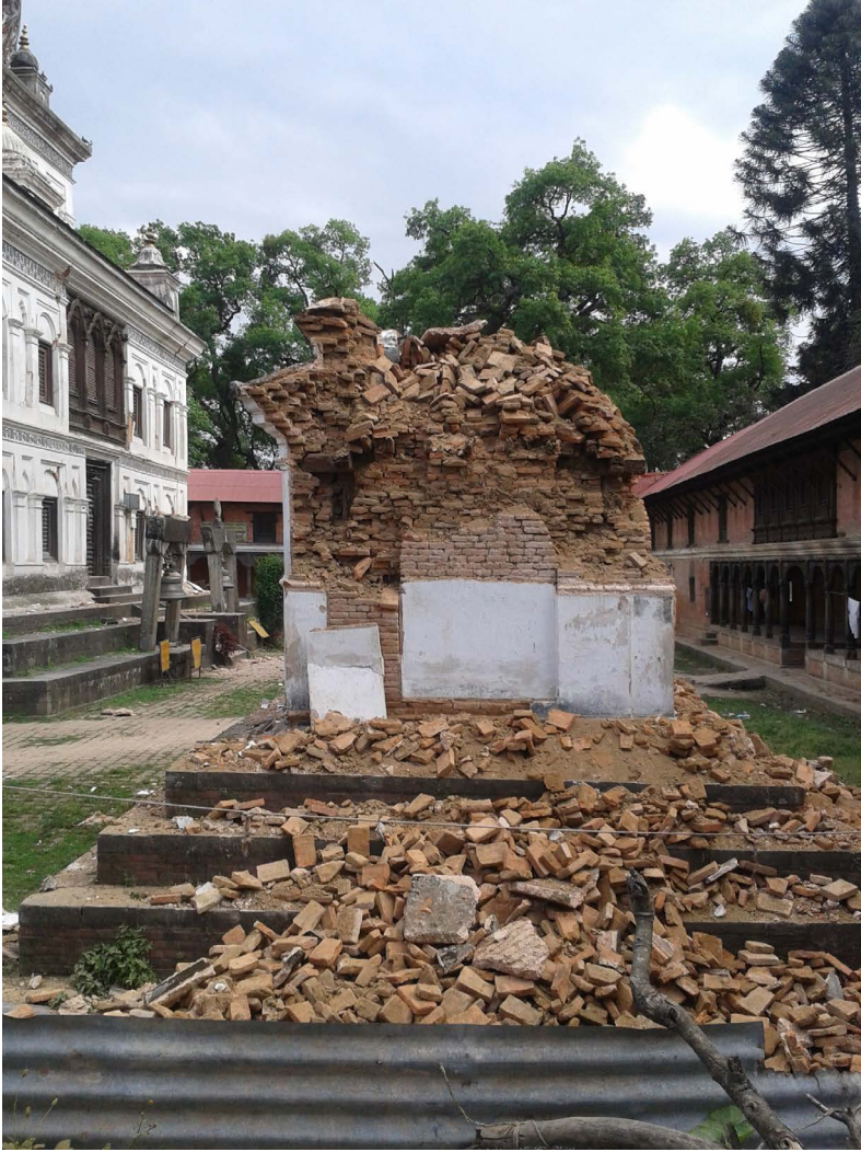
Figure 10. Brick shrine at Pashupati displaying complete masonry failure. (Image: Kai Weise)
