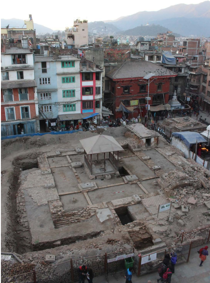
Figure 5. Uncovering the foundations, brick piers and later cross-walls, which formed a mandala, of the Kashtmandap during excavations in 2016. (Image: Durham UNESCO Chair)
